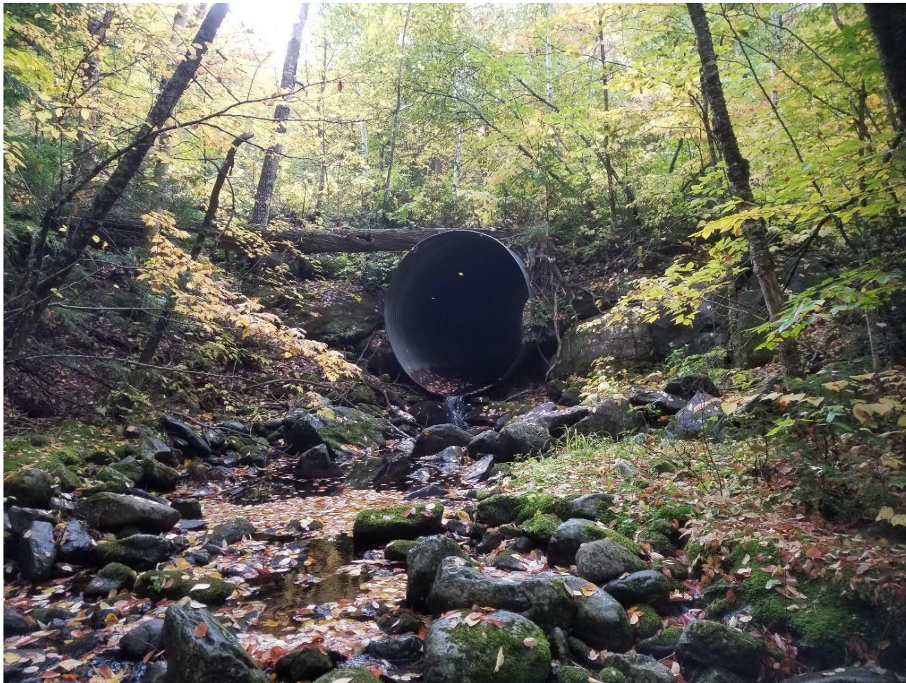
Figure 2. Existing perched culvert outlet at Henderson Brook on the Katahdin Ironworks Road.
